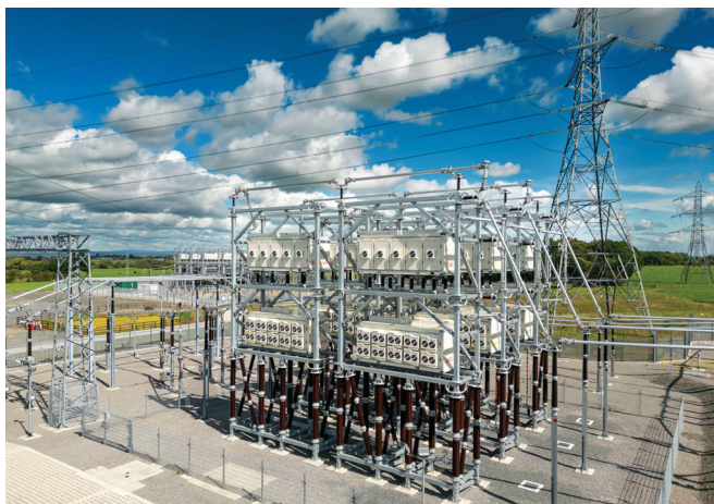
Figure 7. SSSC at National Grid,UK (Smartwires)
