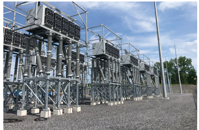
Figure 6. APFC device at Central Hudson,USA (Smartwires)
