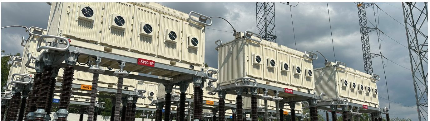
Figure 5. APFC device installed by ISA TRANSELCA, Colombia (Smartwires)
